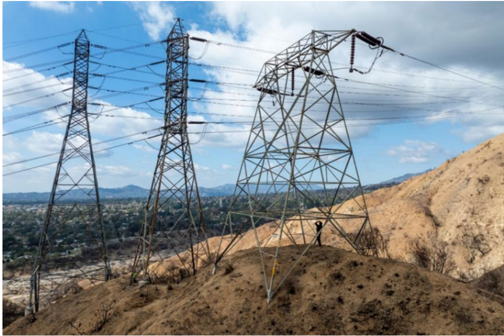
4 5 6 7 8 9 10 11 12 13 14 15 Image 8: SCE Transmission Towers and Electrical Lines (Photo Taken February 11, 2025).
