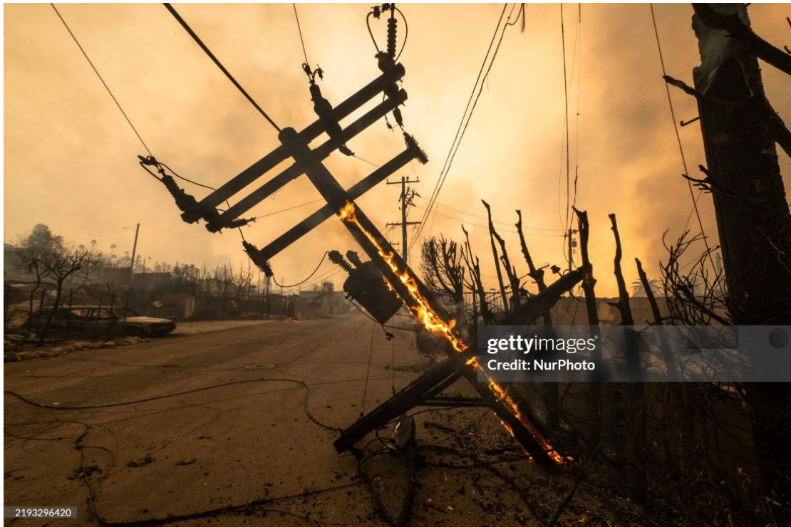
24 Image 13: The Eaton Fire Burns a Utility Pole in Altadena (Photo Taken on January 8, 2025).
